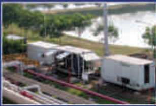
SBU: Tank Sludge Treatment Plant at Cairn Energy India Pte Ltd. at Rajamundry
